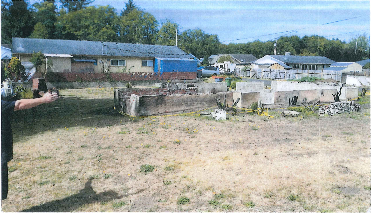
Photo 4: The foundation of the demolished dwelling. The new dwelling will be at this location.
