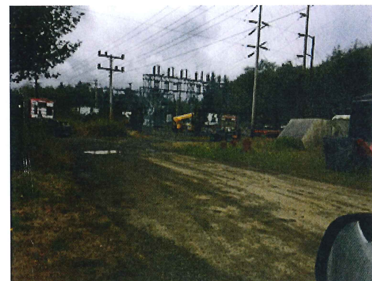
Power Substation at South End of SE Jetty
