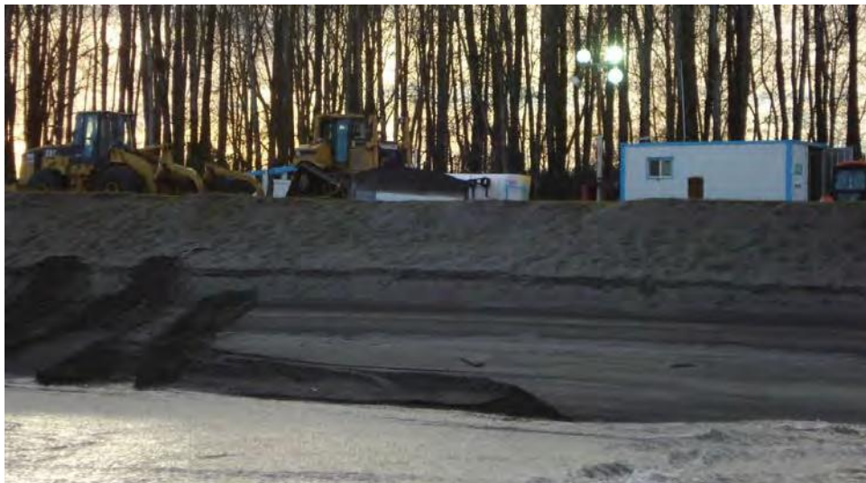
Figure 9: Staging equipment on top of the bank at Sand Island Shoreline Placement Site
