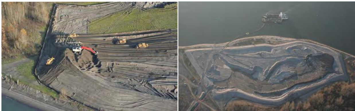
Figure 4: Site preparations and dike building for placement of dredged materials (at Northport).
