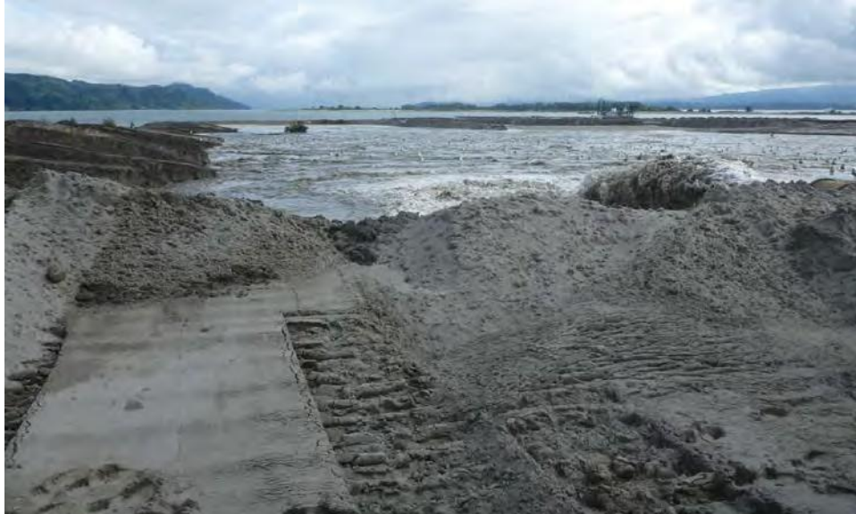
Figure 13: Active discharge of sand and water dredged material slurry at Rice Island Upland Site
