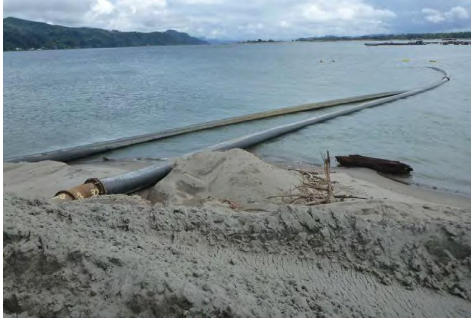
Figure 8: Outfall pipes returning water back to river after dredged material has settled out, Rice Island
